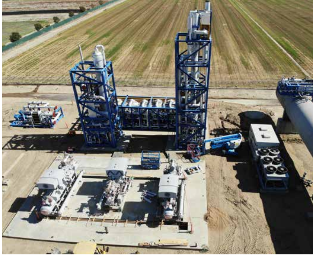
The raw gas for the CO 2 plant in Keyes, California, is extracted from local sources and then purified.
